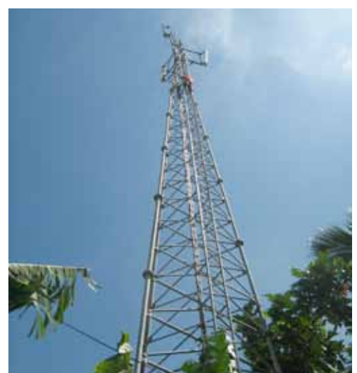
Placing of Radio antenna on towers to get wide radio signal coverage.
