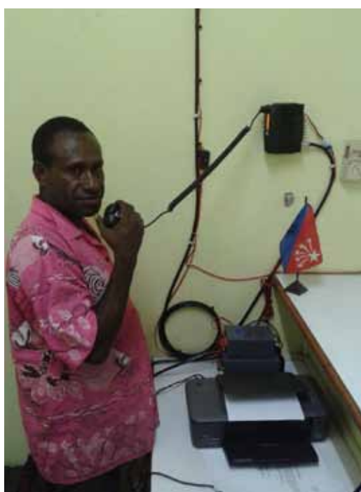
Newly installed VHF radio at Konedobu.
