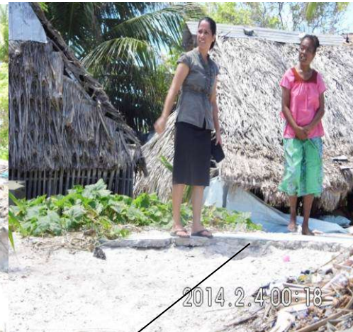
Old cement foundation, broken after the king tides.
