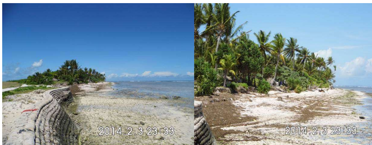
Figure 10: Side view of KAP II seawall. A number of trees had fallen over due to the king tides.
