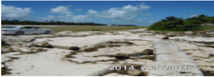
Figure 11: Eroded end and interior of the KAP seawall.
