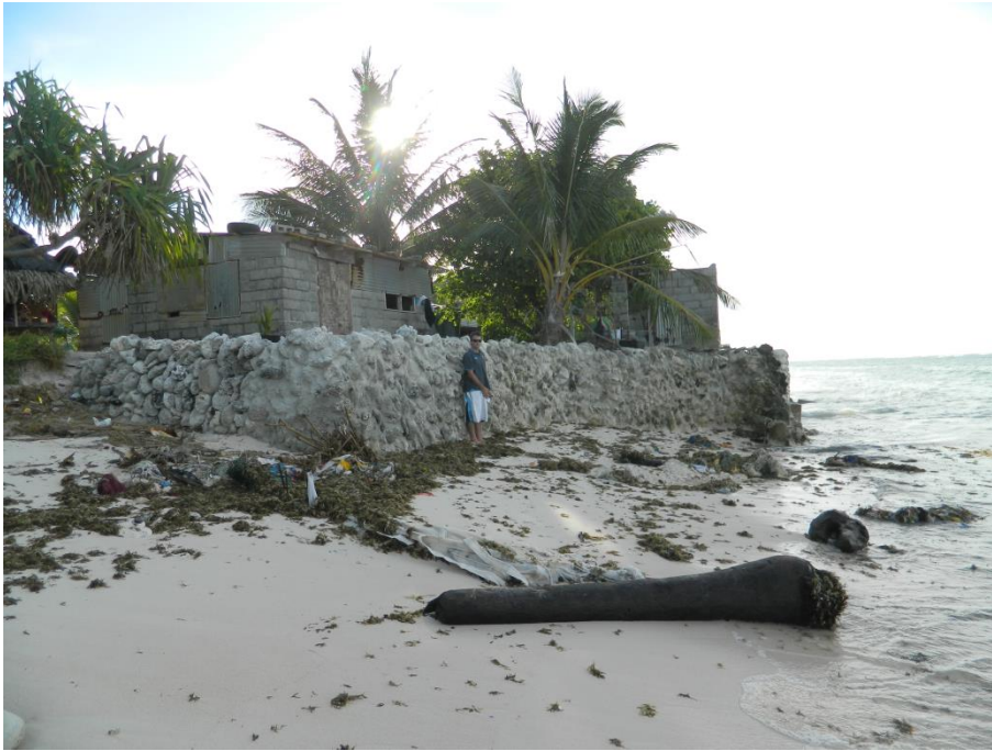
Figure 23: A seawall structure at Bonriki. Vertical hard structures such as these can lead to scour of the beach and interrupt longshore sediment transport, which can lead to erosion along the adjacent shoreline
