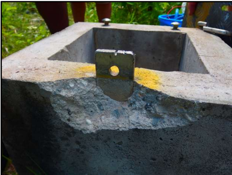
Figure 17: BN2B with the surveyed reference point identified by a notch in the locking lug of the monitoring box. (Damaged monitoring boxes were repaired as part of the project rehabilitation work).
