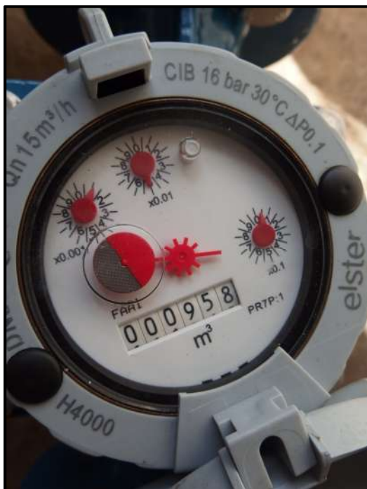
Figure 25: A 50-mm Kent Elster H400 flow meter reading 958.051 \text{ m}^3 .
