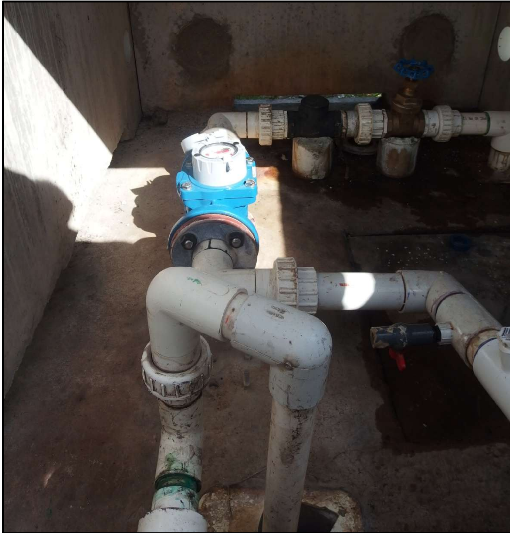
Figure 23: Replacement flow meter installed in gallery 15.
